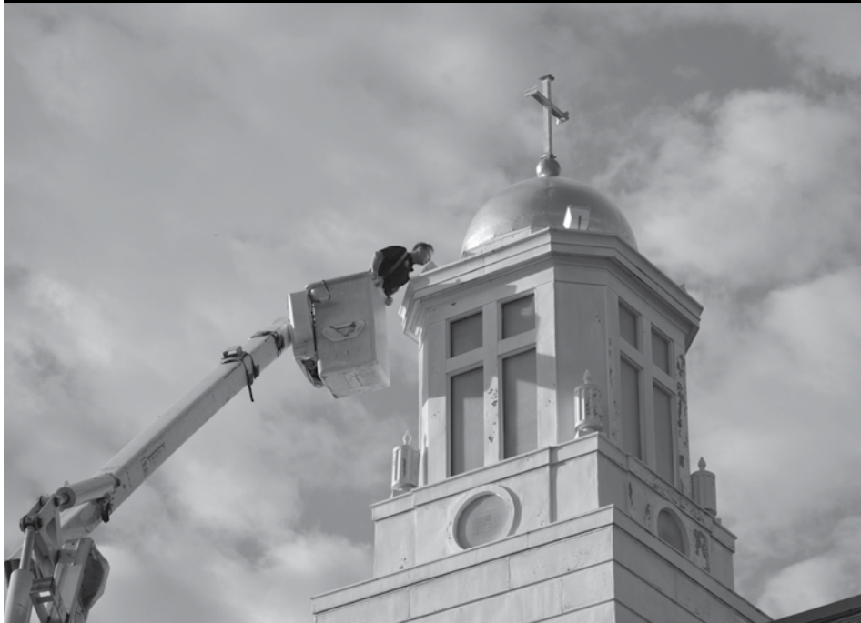
Electrician Harvey Sullivan installs new LED bulbs on the gold dome atop the Collegiate Church of Christ the Teacher Oct. 19. The new bulbs are more environmentally friendly and last longer than the incandescent bulbs that were being replaced.
